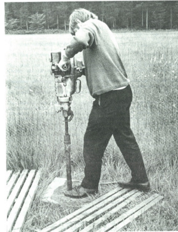
Above: petrol driven Atlas Copco mechanical hammer being used to drive in an access tube.
